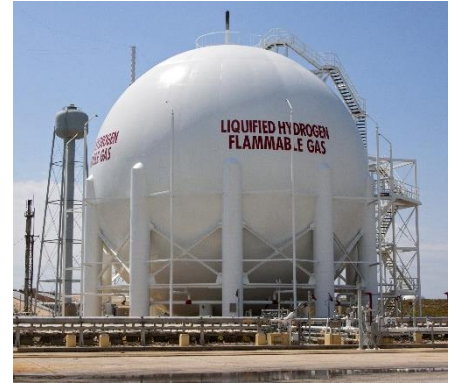
Figure 17. NASA's liquid hydrogen storage tank [58]
